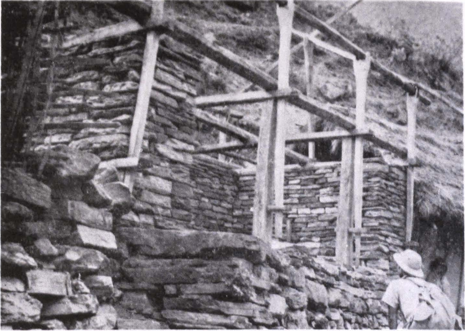
Fig. 74. A house under construction—1. Note the unique technique for supporting beams. At Murali Bang. April, 1953. Photo. by J. Kawakita
